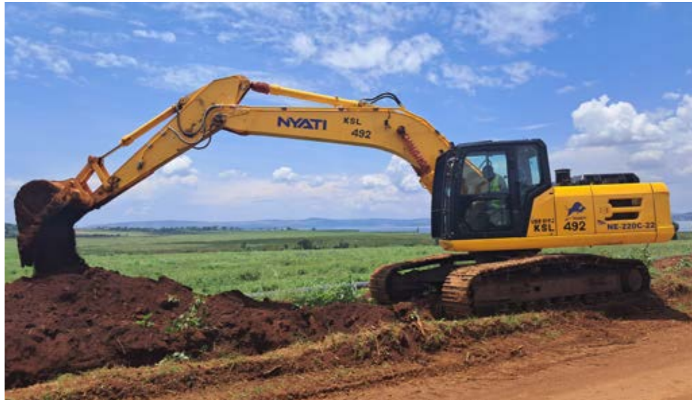
Excavation to place water pipes. Below right, joining HDPE pipes using the butt welding method. Below left, a completed booster pump station at Kakira estate
